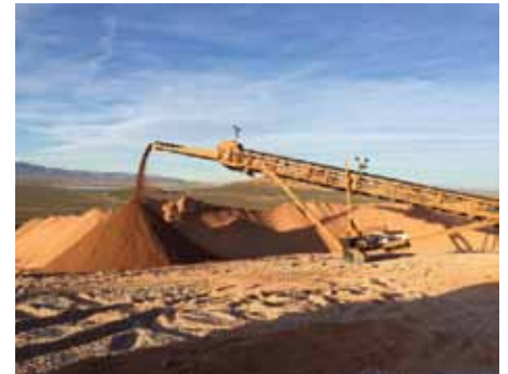
Stacking ore on the heap leach pad at the Soledad Mountain gold-silver mine. Photo courtesy Golden Queen Mining Co. Ltd.
