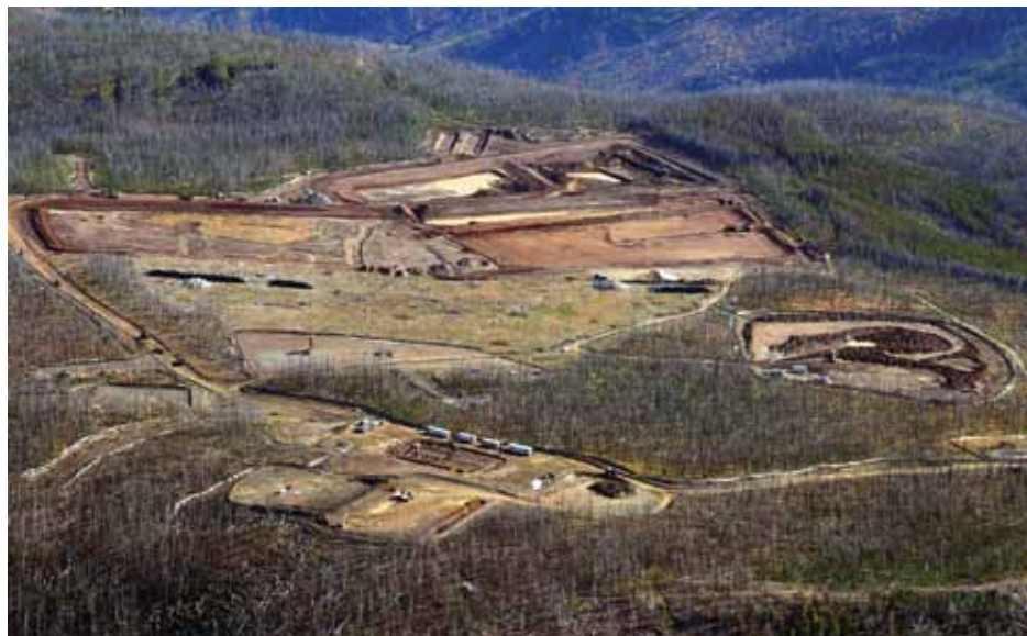
The Idaho Cobalt Project mill and concentrator pads, tailings waste storage facility and water management ponds' earthworks. Photo courtesy Formation Metals Inc.
